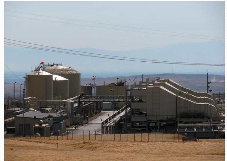
Cyclic steaming cogeneration plant
