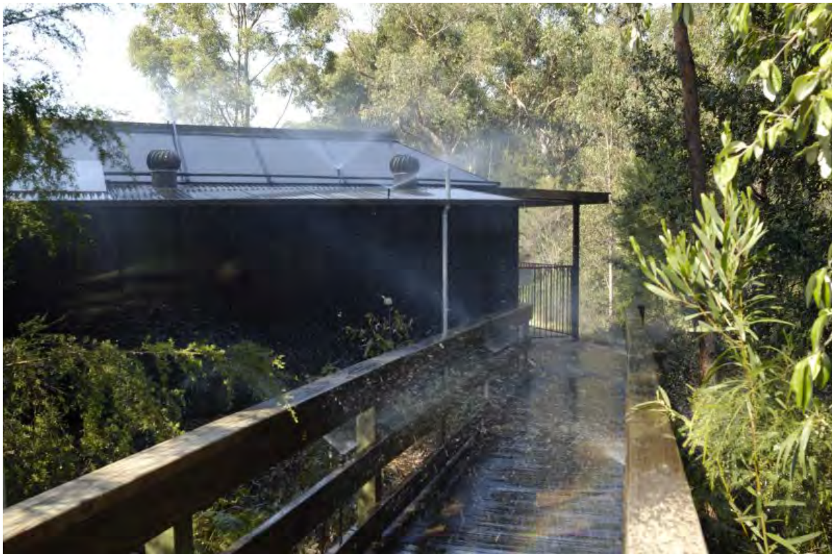
Figure 7. External Sprinklers. As a wildfire approaches, external sprinklers wet the structure at risk, the surrounding environment, and increase the local humidity to prevent ignition. Photo: A conference center in New South Wales, Australia.
