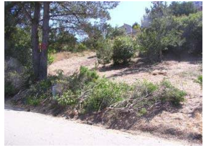
The right way: Deftly removed plants, without the destructive intrusion of big machinery. Chipping was done within a week.
