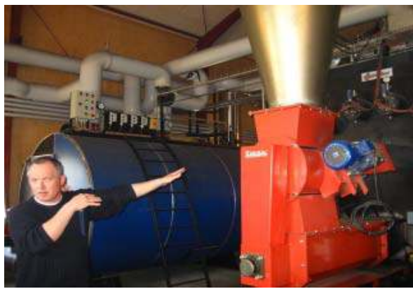
Soren Hermansen with straw biomass district heating burner on Samsøe.
