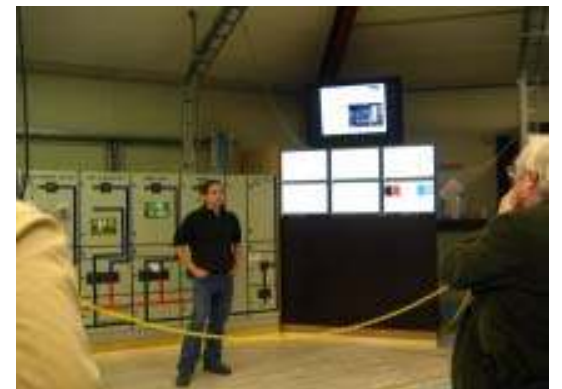
Oliver Gehrke of RISO National Laboratory in front of electrical panels receiving data from renewable energy sources. At right is Dr. Gordon Ashley.
