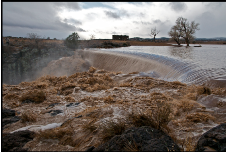
Figure 6. Winter storm flood flow overtopping Sullivan Dam (January 21, 2010). Photo credit: Gary Beverly
