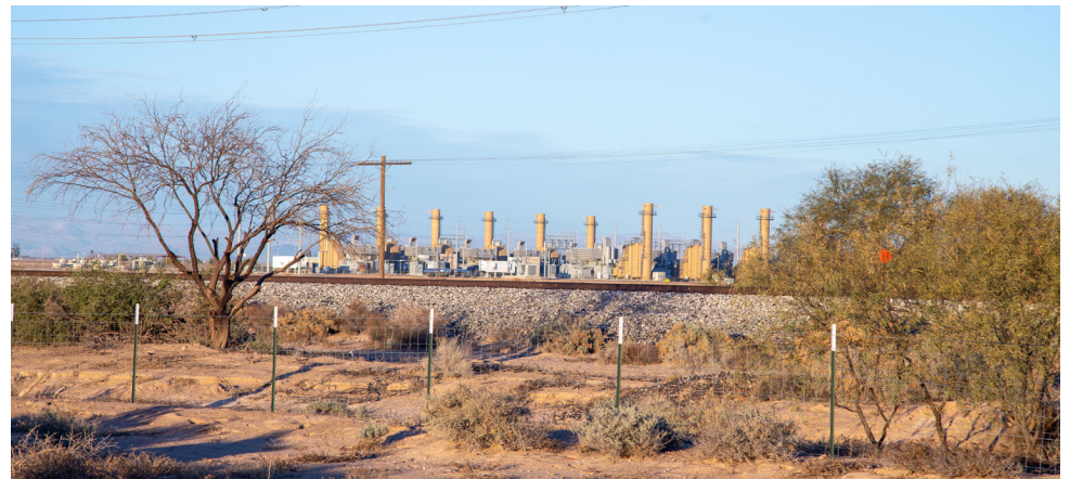
Coolidge Generating Station photo by Caryn Potter
